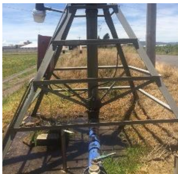
Figure 8 Main pipe and stopcock
